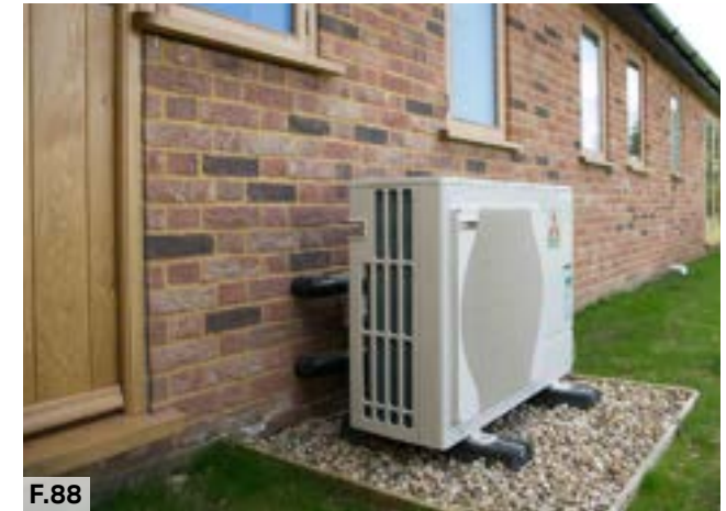
Figure 88: Air source heat pump unit hidden out of view at the rear / side elevation of a building
